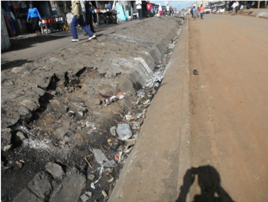
Photo 2 Even with improved drainage, the challenges of erosion and contamination continue.
