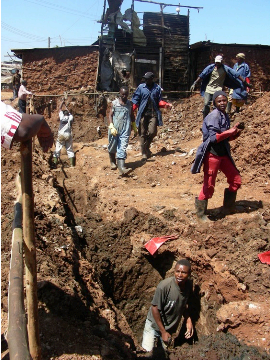
Photo 6 Manual work employs people from the community, but is slower and more difficult to plan and manage than a job done by a mechanical digger.
